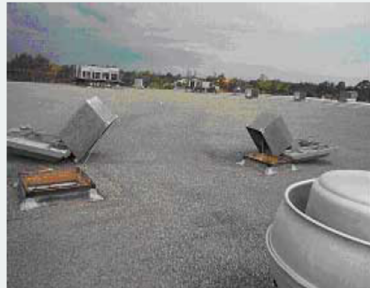
Inadequate attachment provided
