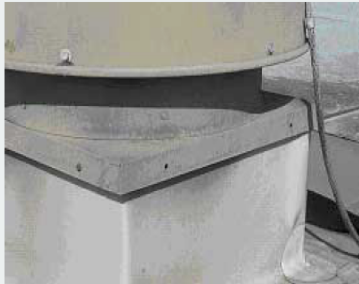
Roof top equipment missing screws
